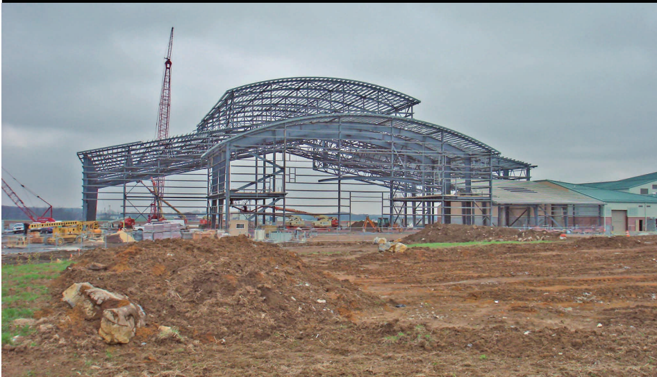
West Virginia Air National Guard C-5 Corrosion Control Hangar Martinsburg, West Virginia
